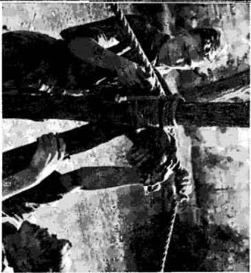
Make the pads of two pieces of burlap. Place in the two shear crotches. Lay all three ropes into the crotches. Lead ends of the foot rope in two turns around the first stakes on each side of river. Then tie them with two half hitches, pulling rope tight.
